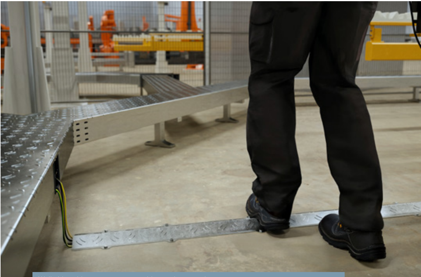
Walkable cable cover to protect cables on the ground.
